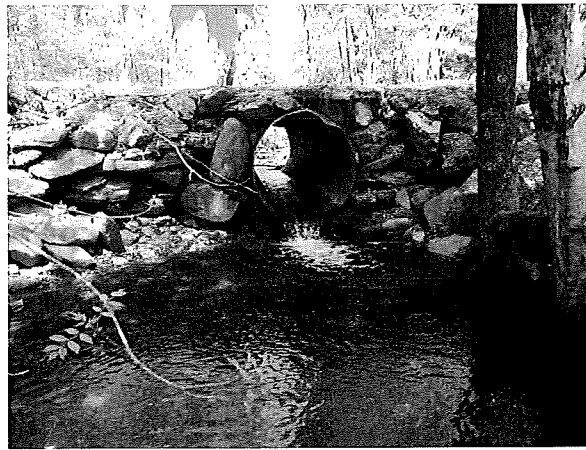
Photo 2: Perched culvert outlet with collapsing headwall.
