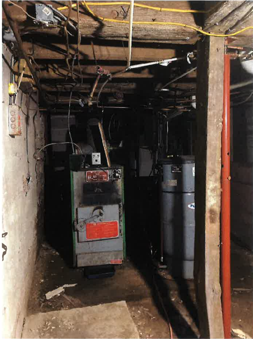
Pigeon House: Basement utilities.
