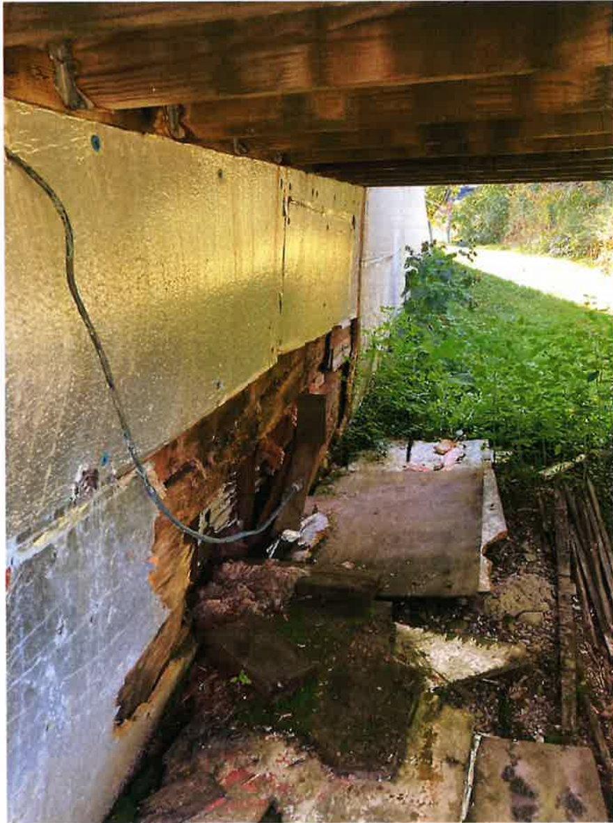
Pigeon House: failed rear wooden basement wall
